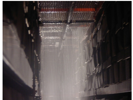
Sprinkler Activation High Pile Storage
