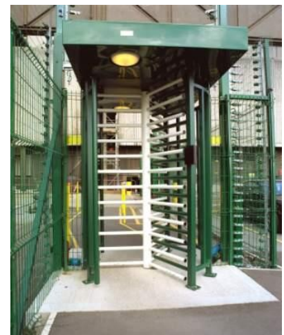
Walk through portal
